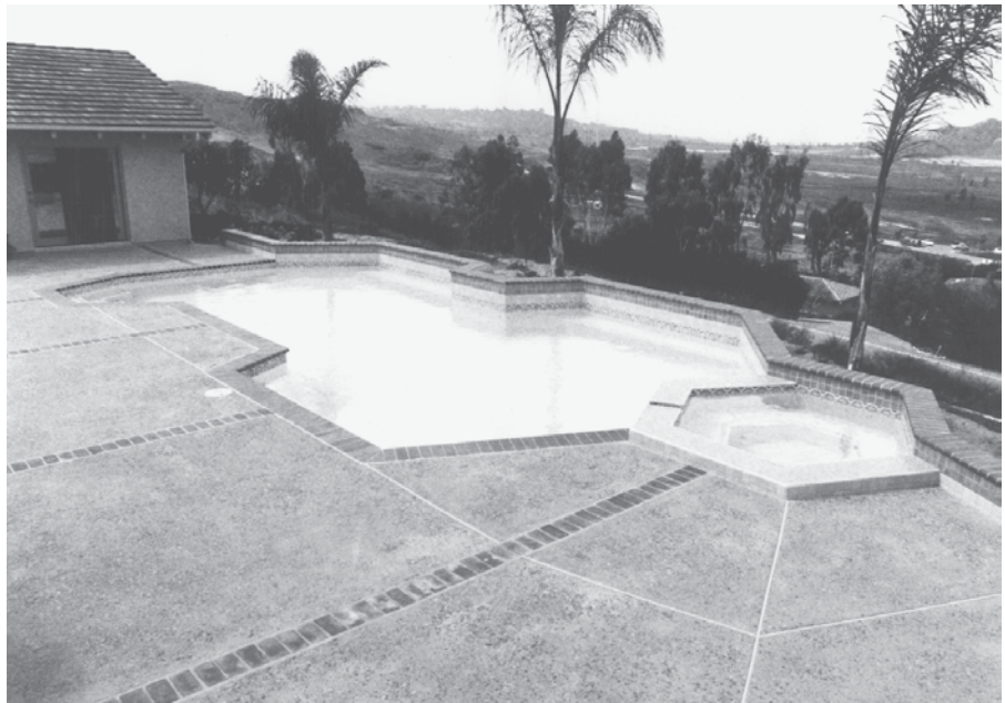
FIGURE 1-21 Typical pool coping, deck, and expansion joints. Questar Pools and Spas, Escondido, Calif.
