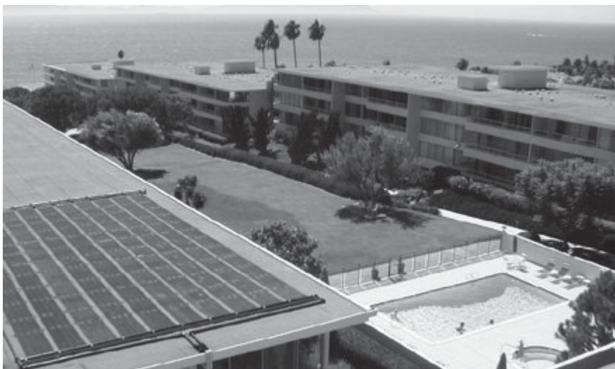
FIGURE 3-7C Solar heating on rooftop.
