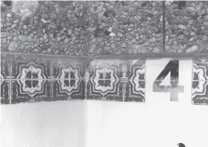
FIGURE 1-20 Scale deposits on tile.
