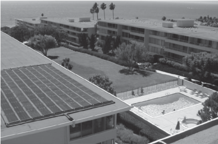
FIGURE 6-10 Rooftop solar installation. Suntrek Industries.
