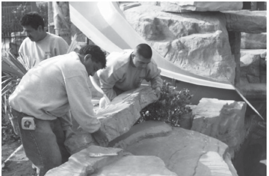
FIGURE 11-3 (A) Artificial rockscape: waterfall; (B) artificial rockscape: concealed equipment area. www.ricorock.com , by Rock Formations, Inc.
