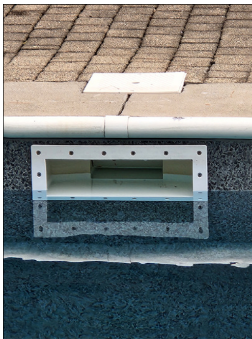
FIGURE 3-1: This inground pool skimmer has a water level about an inch too low.
