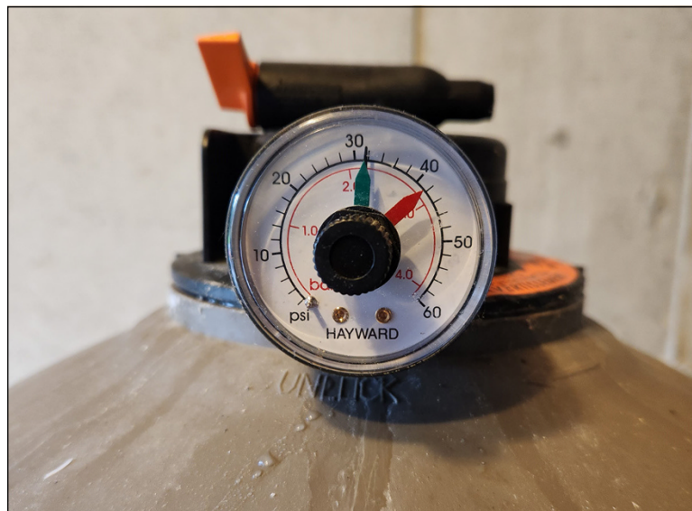
FIGURE 3-9: A pressure gauge with start (light) and time-to-clean (dark) arrows.
