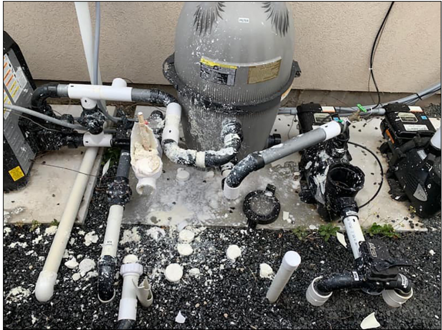
FIGURE 3-3: A chlorinator that exploded because of cal hypo-based chlorine tablets.
