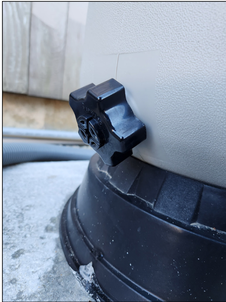
FIGURE 4-3: The drain cap on a sand filter.
